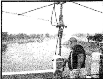
Atop the roof 25 feet up, Alexander Hilliard, W4GMM (AFA2FL), of Memphis checks the beam mounting of the Corps of Engineers station. Photo by James Pogue, KH2AR.
